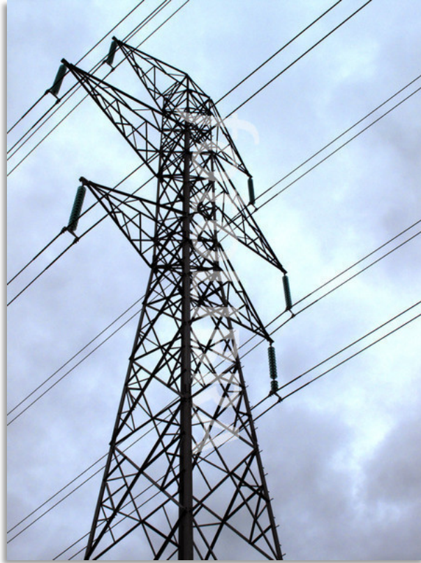
Figure 6-1: Typical Electrical Pylon
