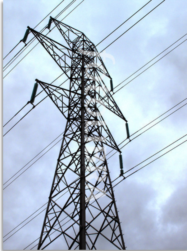
Figure 6-1: Typical Electrical Pylon
